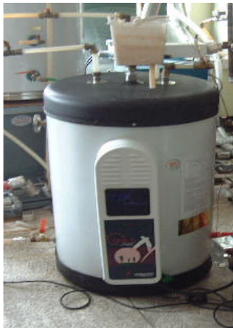
Fig. 2 The front of the midnight electric boiler.
