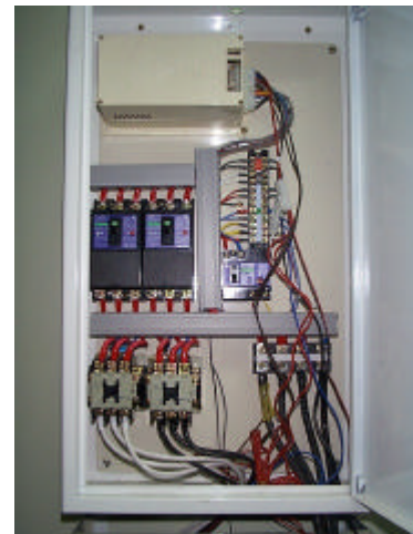
Fig. 4 Electric supply plate, the midnight electric boiler.
