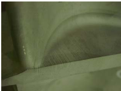
Fig. 6 Typical platform crazy cracks
