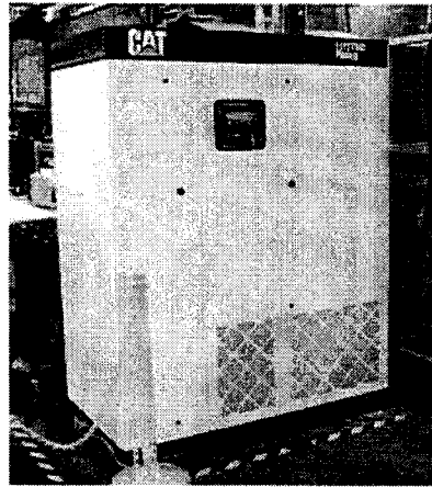
Figure 8. CAT UPS shown installed at the EPRI PEAC testing facility
