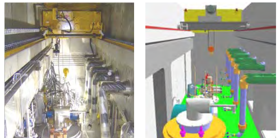
Fig. 1 The Real and Virtual ACP Demonstration Facility
