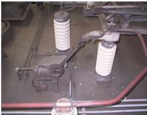
(b) Emergency ground switch weld
