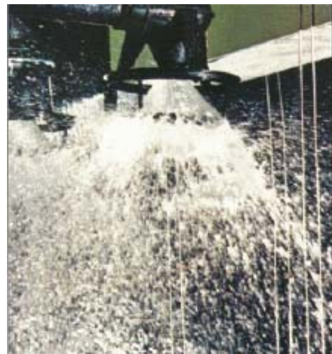
Figure 5 Water distributor nozzles
