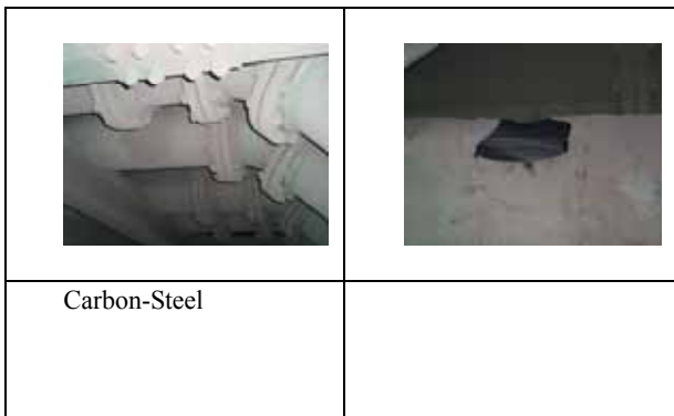
Fig. 1 Abrasion within the curved section of pipe
