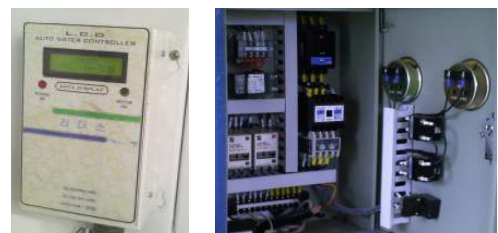
Fig. 6 controller for water supply(pump)
