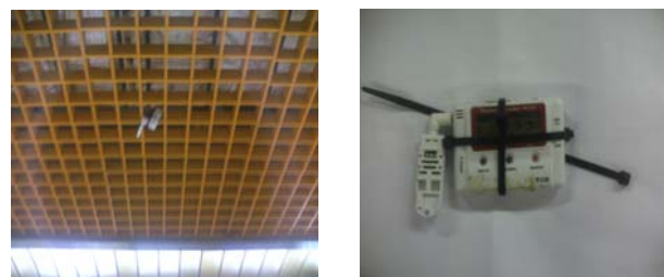
Fig.1 Platform temperature, humidity measuring device
