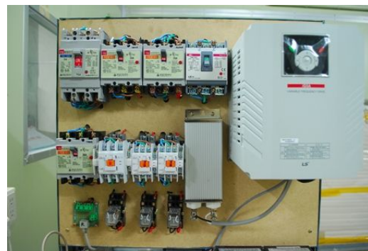
Fig. 4 View of control panel
