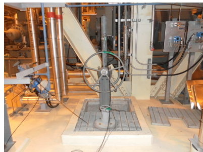
Fig.1 Yoke part of isolation valve damaged
