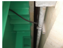
(b) Before installation
