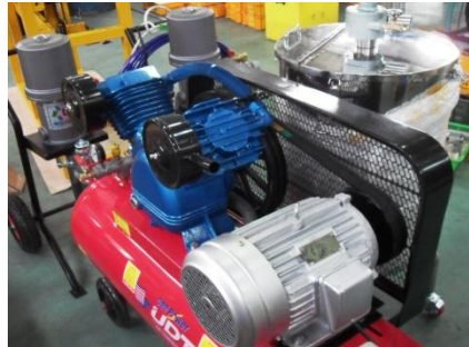
Fig. 4 General view of utility system
