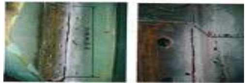
Fig. 1 Damages of crossbeam
