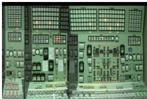
Fig. 1 Main control board
