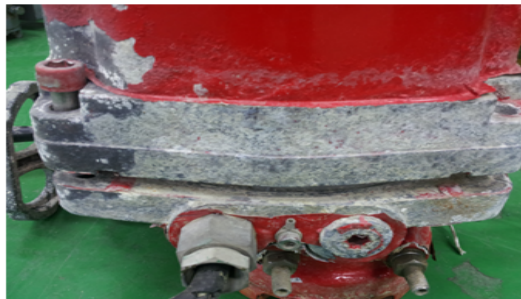
Fig. 1 surface corrosion faulty of marine paint coating
