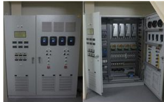
Fig. 3. Control panel of C-1 drive synch system.
