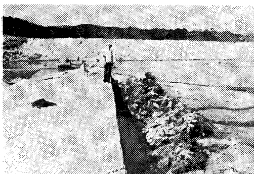
Fig. 7. The feature of apron and protected river bed destroyed
