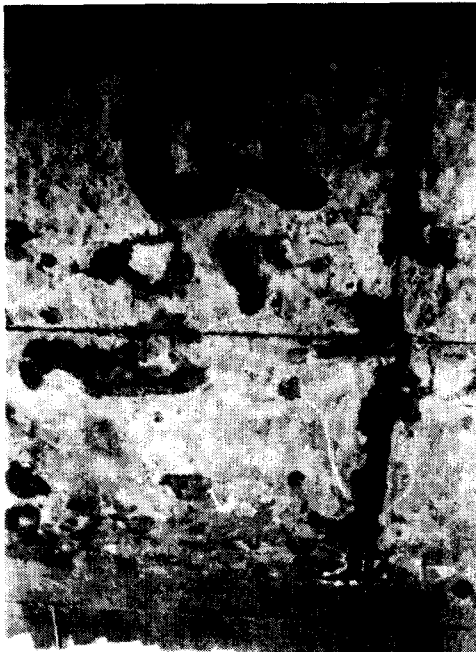
Photo. 4 Pitting in hull
