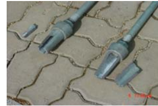
(a) Splice damage
