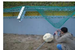
(c) Rockfall protection fence damage(rockfall energy=12.3kJ)
