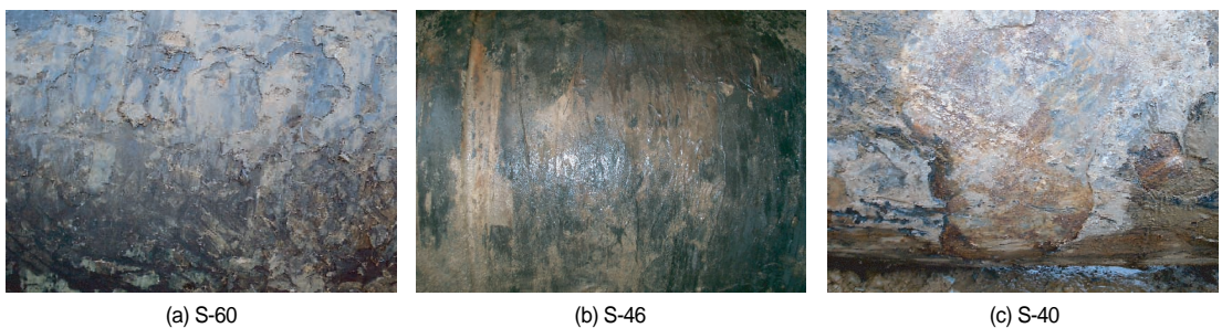
Fig. 3. Examples of Internal lining or coating damages of large water mains.
