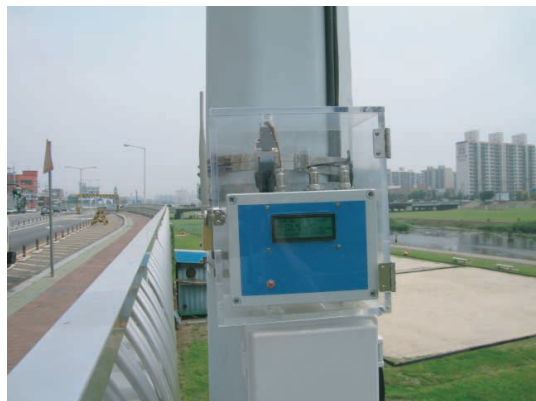
Fig. 2-b. Water quality data transmission system installed in the study site.
