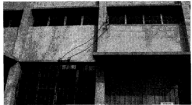
Fig. 6. Low voltage distribution system at lab
