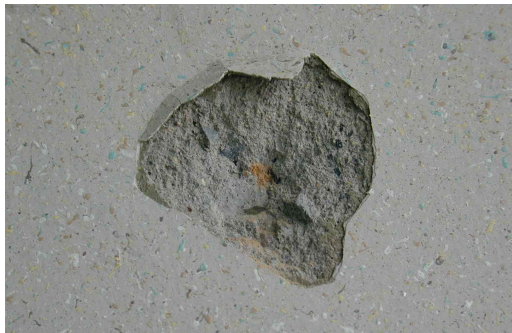
Fig. 1 Example of pop out on concrete surface
