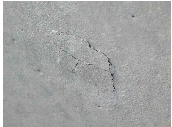
Fig. 11 Example of pop-out on normal-set mortar
