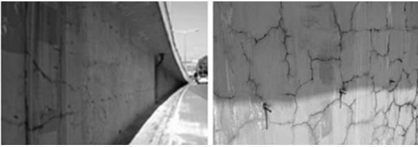
Fig. 1 Seriousness of the crack which occurred in the concrete structure
