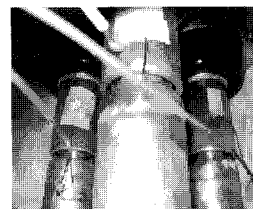
(a) Conductor surface
