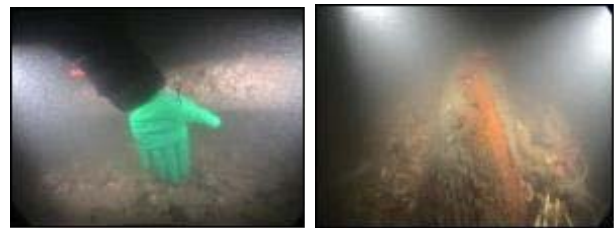
Fig. 7. Damage of submarine cable.
