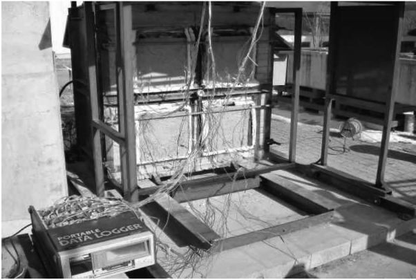
Fig. 5 Measurement of temperatures using data logger
