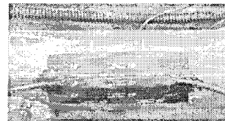
Fig. 4 Sensor attached on pipe
