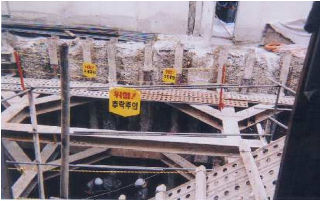
Figure 4. Fall risk and overturn risk of temporary material
