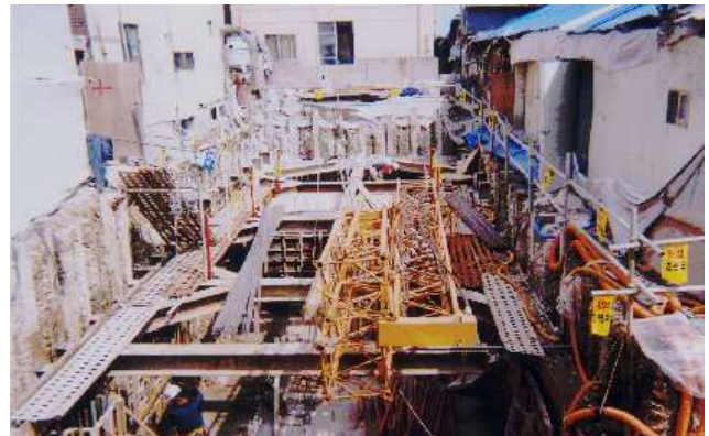
Figure 3. Situation of dangerous article neglecter
