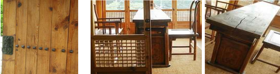
Fig. 4. Images of Shake and Gnarl shown on the Hansam DBEW Design Center Gate and Wooden Tables in a Lounge in the Building
