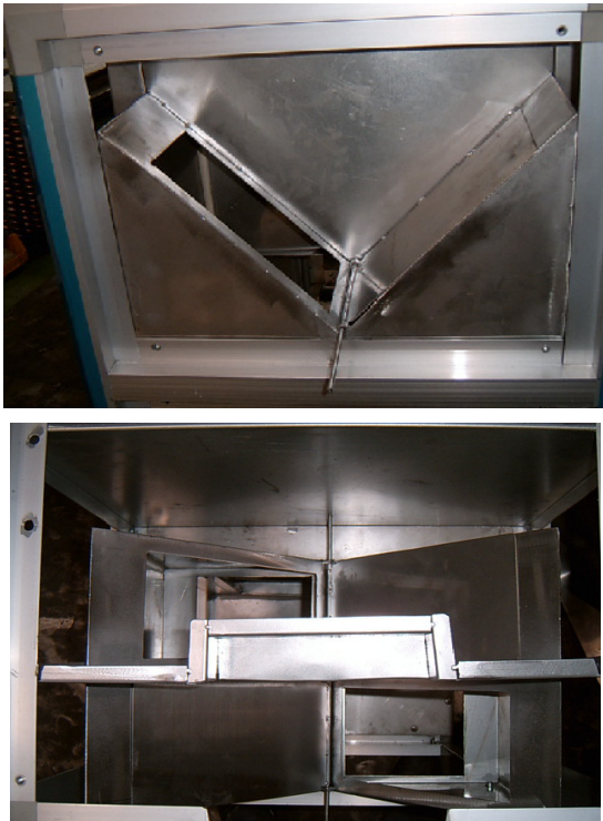
Photo. 2 An installed air shifter.
