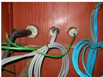
(c) cable hole in manhole
