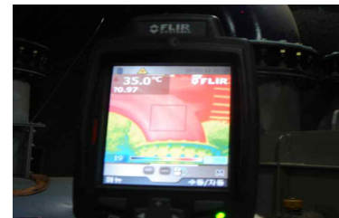
Fig. 4 Diagnosis of blower facility
