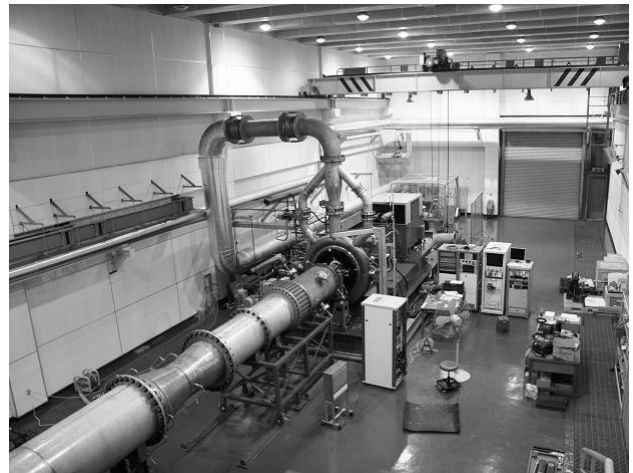
Fig. 7. KARI Compressor Test Facility
