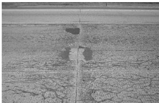
(a) Map cracking
