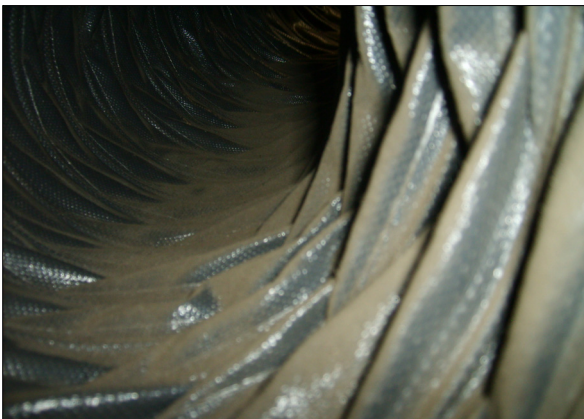
Fig. 2 Pollution in ducts.
