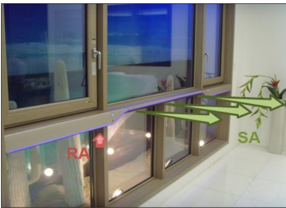
Fig. 1 Thin line type ventilator installed on a window frame.
