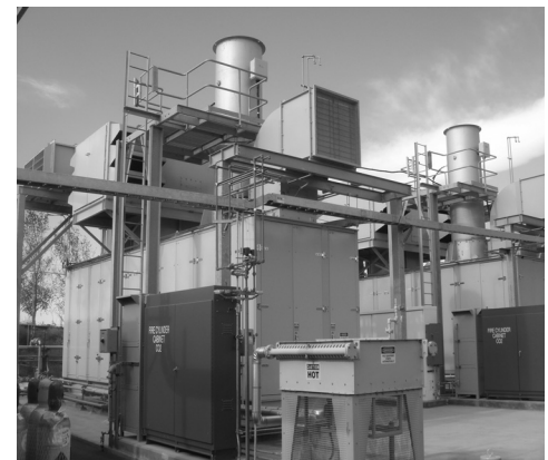
Fig. 2 4.6MW-CLASS Biogas turbine & Fuel pretreatment system (10) (Calabasas, CA, USA)
