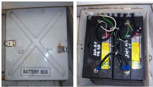
Figure 6: Photograph of battery case
