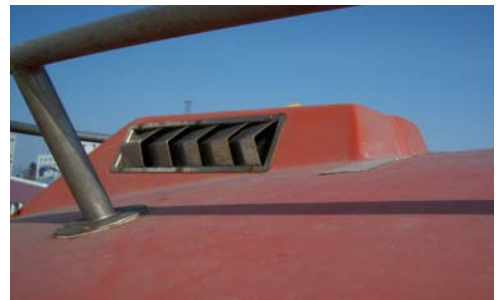
Figure 8: Photograph of lifeboat vent
