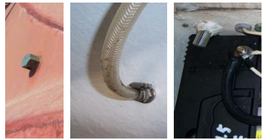
Figure 7: Photograph of battery vent
