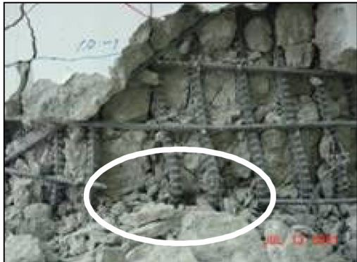
Fig. 2 Failure by fracture of transverse steel 9)
