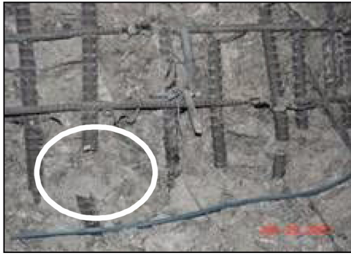
Fig. 1 Failure by fracture of longitudinal steel 9)
