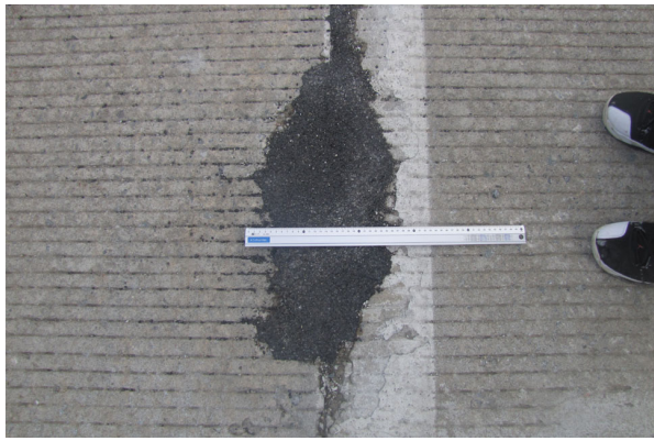
(a) Distress on Longitudinal Tining
