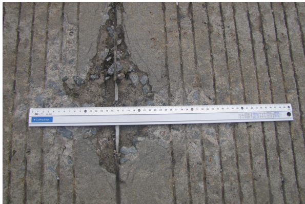
(b) Distress on Transverse Tining
