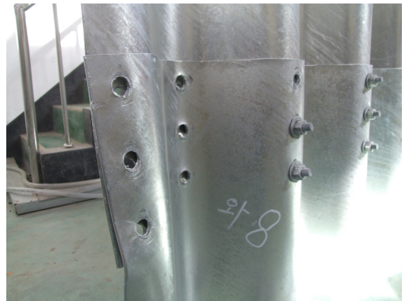
(d) combined failure with bolt shearing and local buckling
