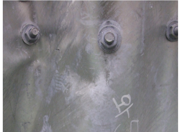
(b) combined failure with plate bearing and local buckling (II)
