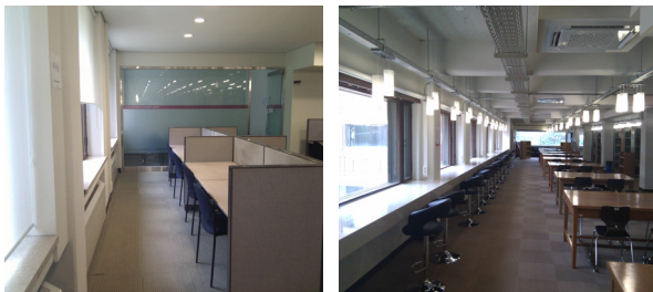
1st floor : fan coil units installed on window-side
