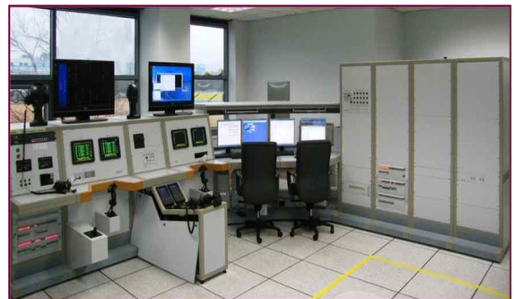
Fig. 9. MEP System Integrated Laboratory
