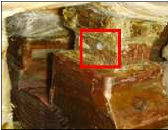
Fig. 10. Water absorption winding due to coolant water leaks
