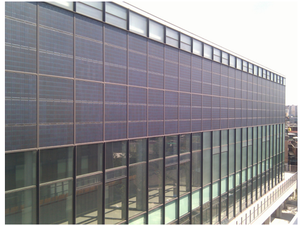
Fig. 2 The BIPV on curtain-wall.
