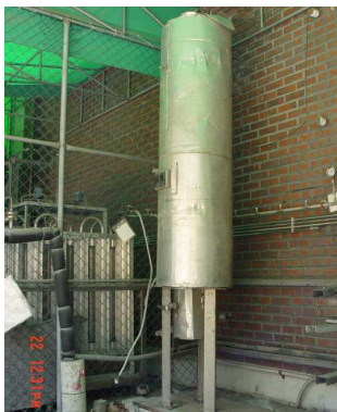
Fig. 2 LN 2 storage tank
