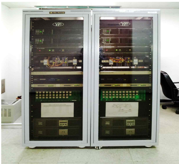
[Fig. 4] Station Control Unit Installed on the Naepan Station
