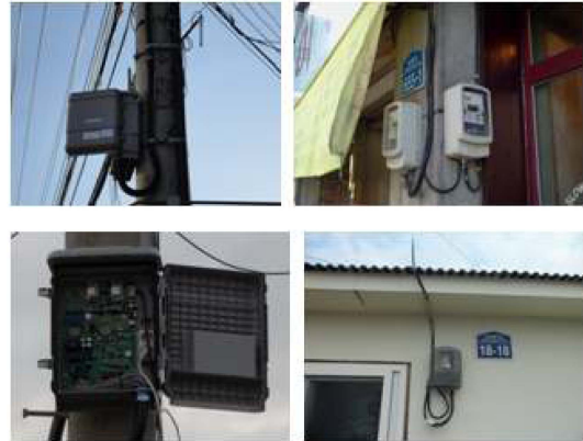
Fig. 9. DCU and electricity-meter for AMR.
