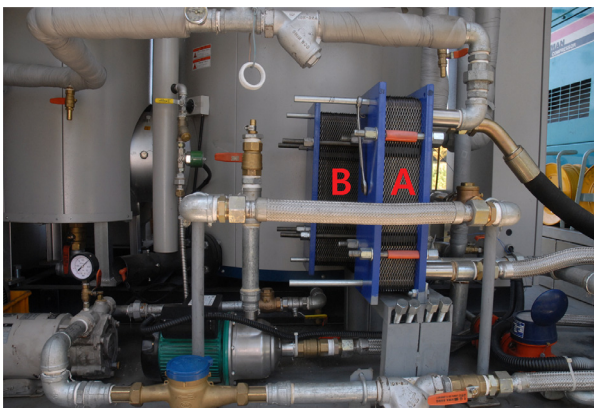
Fig. 3 Photo of the plate heat exchanger.
