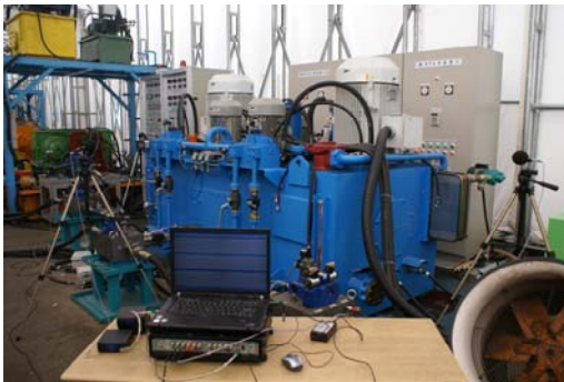
Figure 3: Vertically installed HPU without shield chamber
